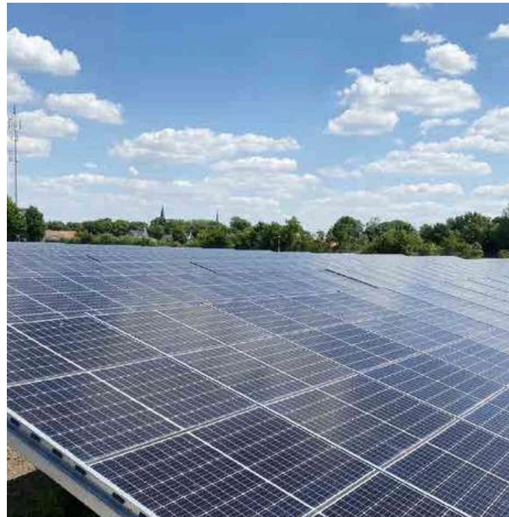
1.16MW The Netherlands
